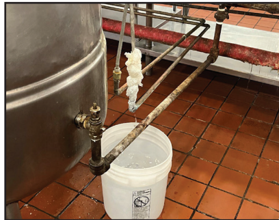
Facility A—Leaking Kitchen Kettle Pipes
