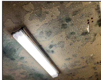
Facility B—Deteriorated Ceiling
