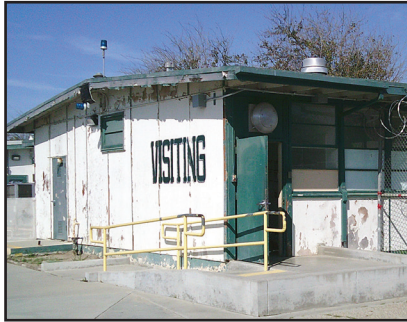
Facility A—Dilapidated Visiting Area
