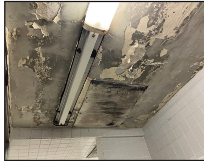
Facility C—Deteriorated Restroom Ceiling
