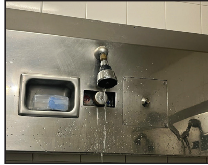
Facility A—Leaking Shower Faucet
