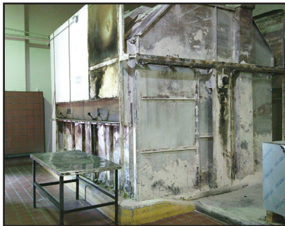
Facility D—Damaged Kitchen Oven
