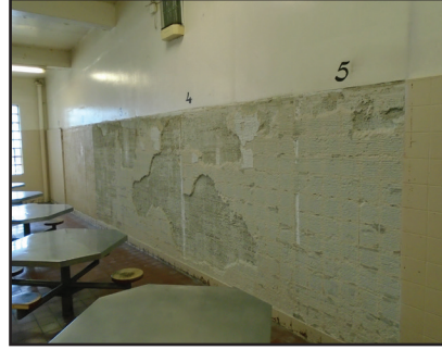
Facility B—Damaged Mess Hall Wall
