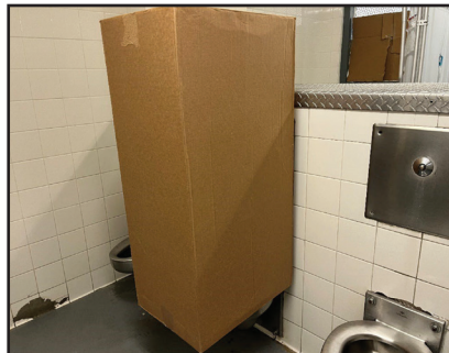
Facility A—Nonfunctional Toilet
