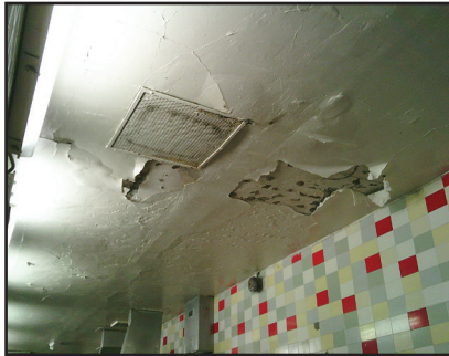
Facility C—Damaged Kitchen Ceiling
